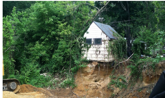
Prior to installation, stream was extremely eroded and threatening surrounding area.
