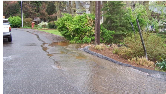
BEFORE: the rain garden, street flooding was common and muddy. Photo Credit: Eloise Ullman
