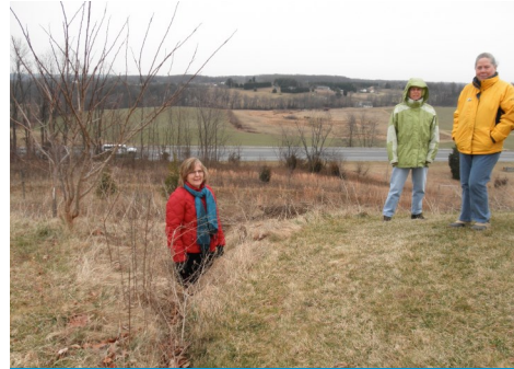
The erosion ditch had gotten so bad it created a safety hazard and was waist deep!
