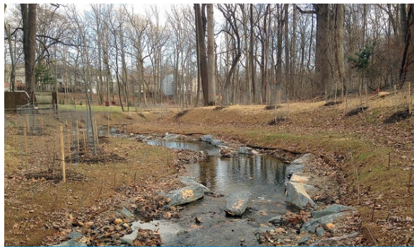
The same area of stream, after restoration Photo credit: Montgomery County DEP
