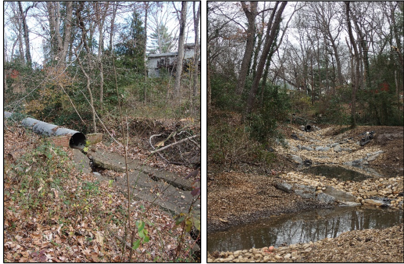
Olde Severna Park Outfall Retrofit: before (left) and after (right). Photos courtesy of Anne Arundel County DPW.
