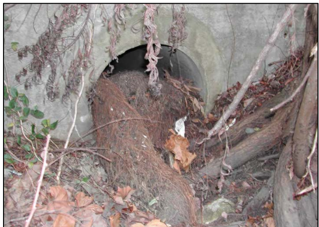
An obstructed outfall in Bowie.
